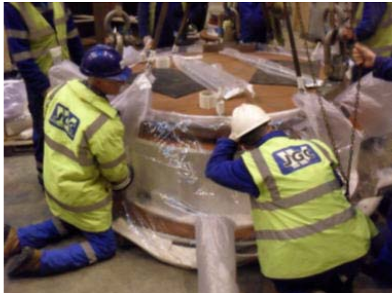
Figure 3 shows a purge bag being fitted to the PCTL upstand during off-site component testing.
