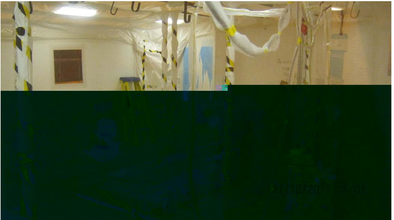
Airline suit worker removing redundant equipment from the former MTR Reprocessing Plant
